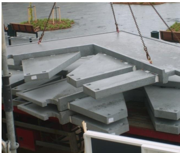
Figure 1: Cantilevered balcony elements ready for installation. The cantilevered flaps are cast monolithically as part of the element for attachment to the building façade.
