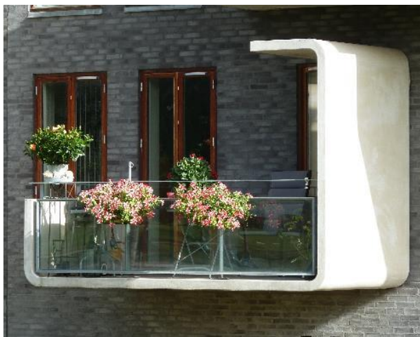
Figure 2: Cantilevered balcony element placed on corbels in the bottom of the deck and with bolted connections transferring tensile forces into the façade from the top of the balcony upstands.
